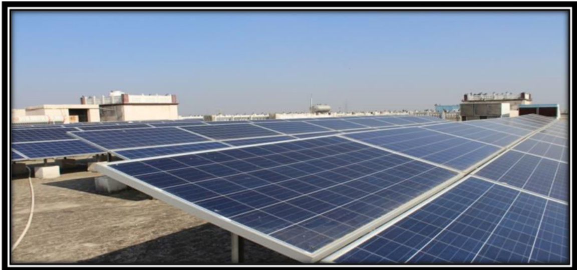
Solar Energy Unit
